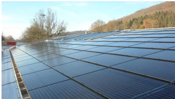
Hausen 1: 30 kWp, 210 m 2
